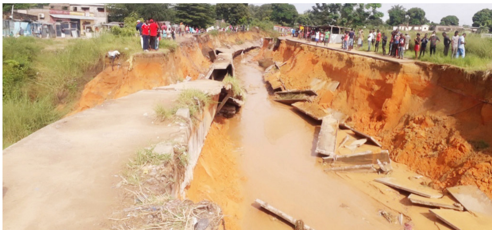
La route effondrée
